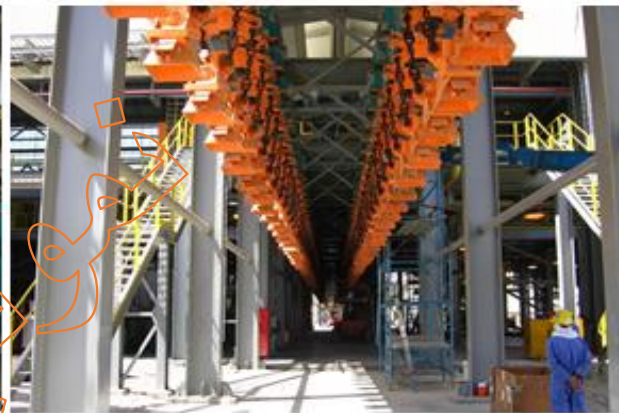
Power & Free conveyor system
